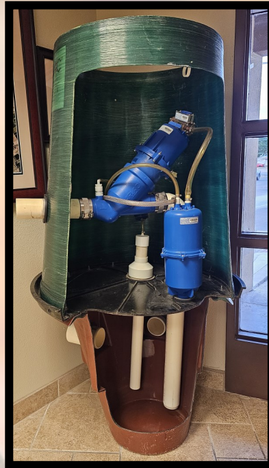
Vacuum Valve Pit
